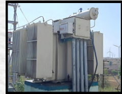
Inverter Duty Transformers
