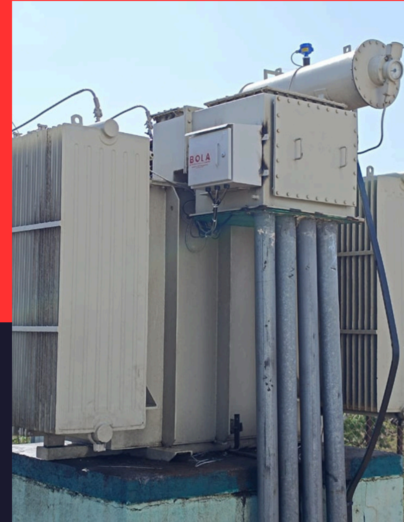
Inverter Duty Transformer
